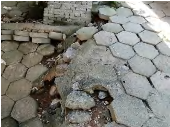
护坡铺砌破损
