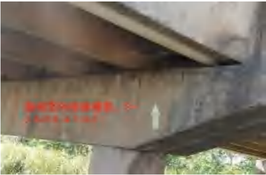
盖梁处钢筋锈胀
