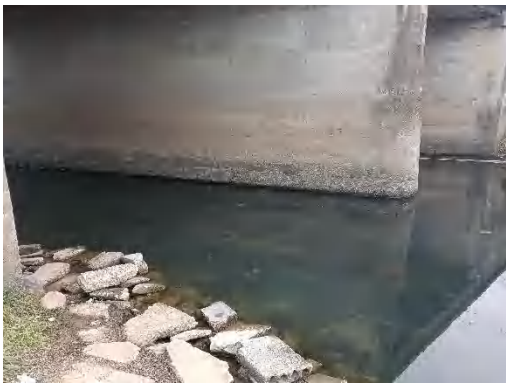
桥墩冲刷露骨
