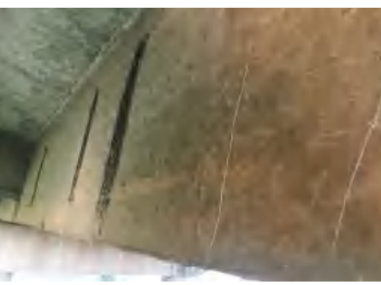
腹板竖向裂缝
