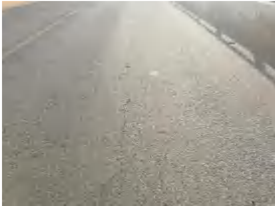
桥面纵向裂缝
