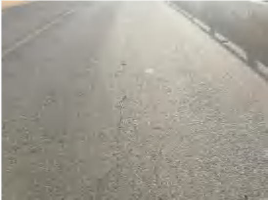
桥面纵向裂缝
